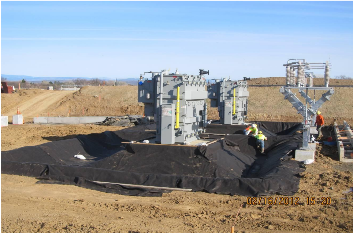
Balfour Beatty installing the oil containment system around the two transformers in the Switchyard.
