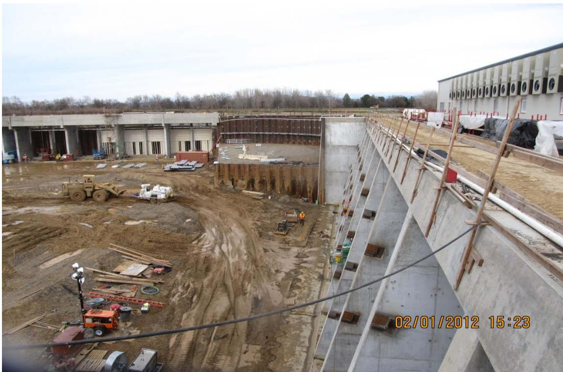
Balfour Beatty welding trash rack supports and tuning baffles at Pumping Plant.
