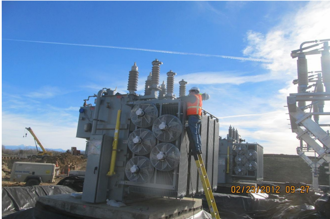
Balfour Beatty subcontractor Virginia Transformers checking the installation of the cooling radiators.
