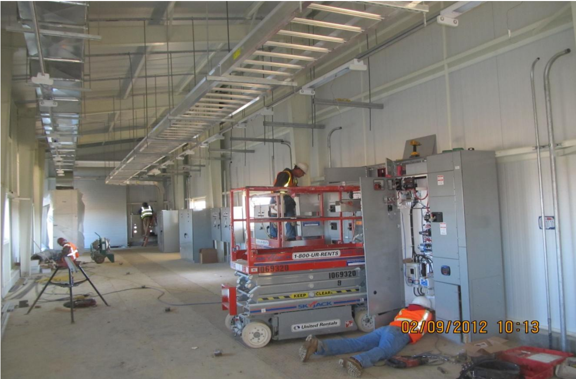
Balfour Beatty subcontractor Central Sierra Electric installing Fish Screen motor control center, conduit, & bracing.
