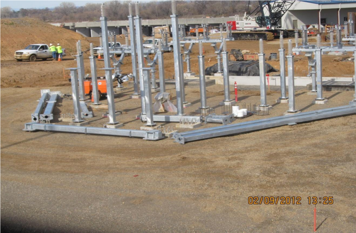
Balfour Beatty erecting Switchyard steel structures with takeoff structure steel staged for erecting.
