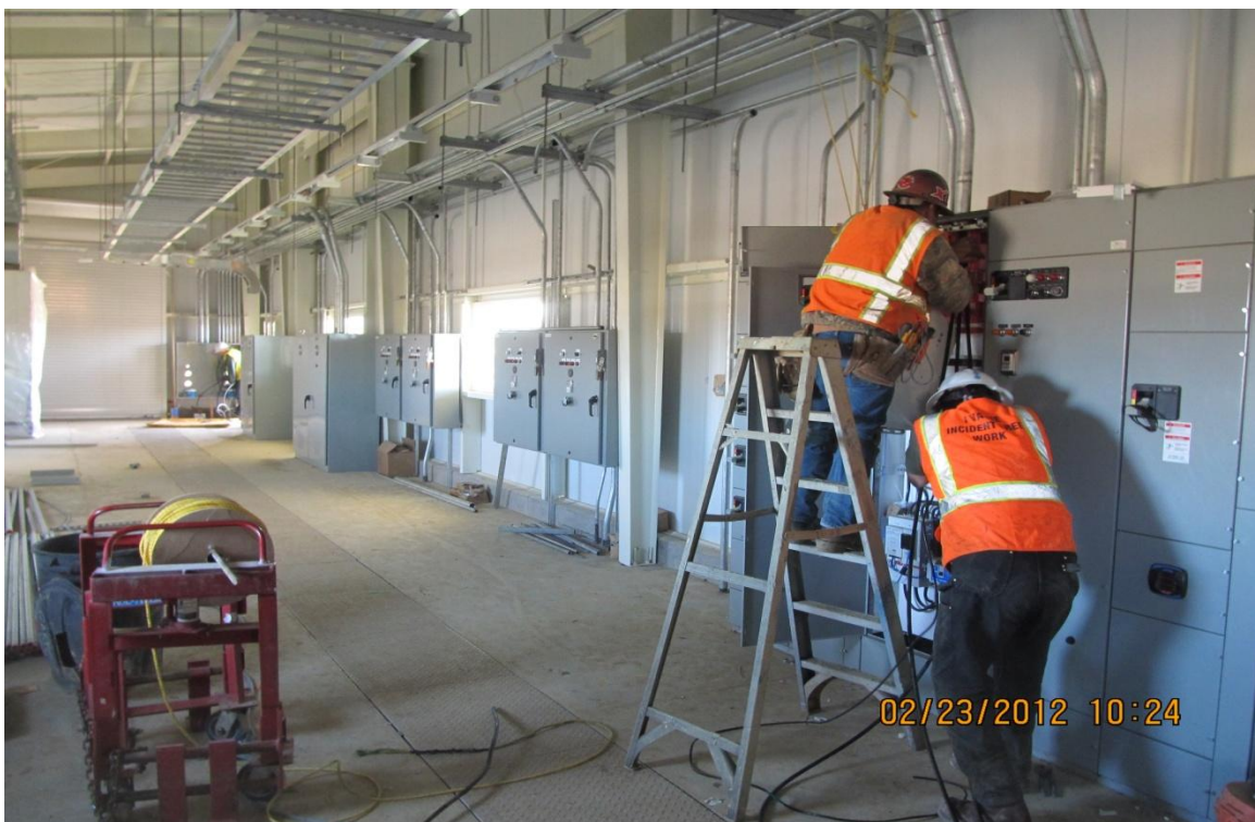
Balfour Beatty subcontractor Central Sierra Electric pulling cables into Fish Screen Motor Control Center
