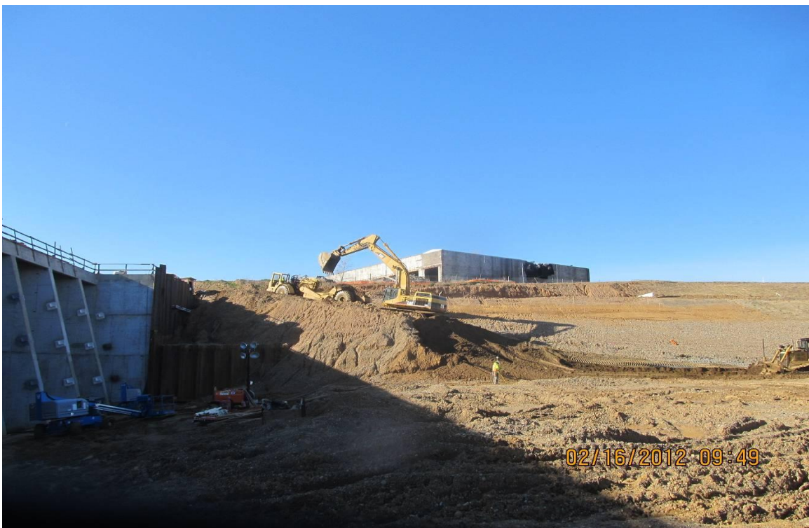
Balfour Beatty subcontractor Meyers Earthwork excavating the forebay upstream side of the Pumping Plant
