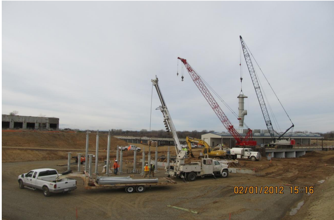
Balfour Beatty subcontractor Harrel's Hi Voltage - foreground. Installation of last 84" pump - background.
